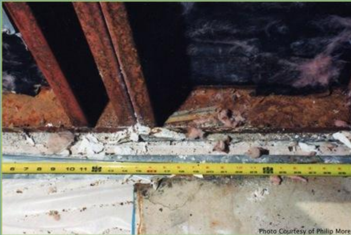
Rusted metal framing and sill plate in a new building
